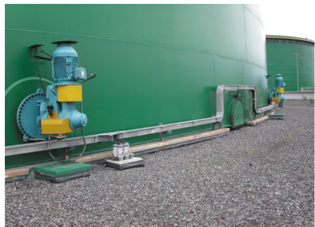
55kW Swivel Gear Mixers installed with Automatic Actuator
