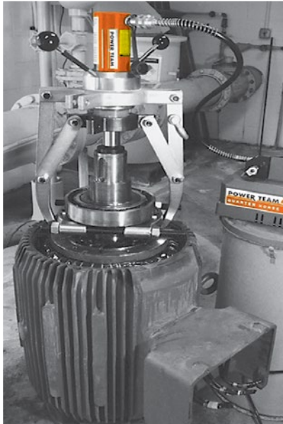
▶ Puller with a bearing pulling attachment was used to take a bearing off a utilities well pump motor.
